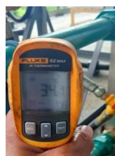
Gambar 10. Temperature Water Outlet Heat Exchanger
