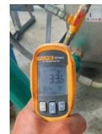
Gambar 8. Temperature Oil Outlet Heat Exchanger
