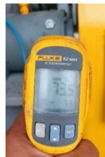
Gambar 5. Temperature Bearing Fan 482-FN5 Motor Side setelah instalasi
