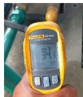
Gambar 7. Temperature Oil Inlet Heat Exchanger
