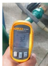
Gambar 9. Temperature Water Inlet Heat Exchanger
